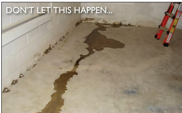
A waterproofing job where Polydrain wasn't used and the concrete replacement floor blocked the weep holes in the wall.
