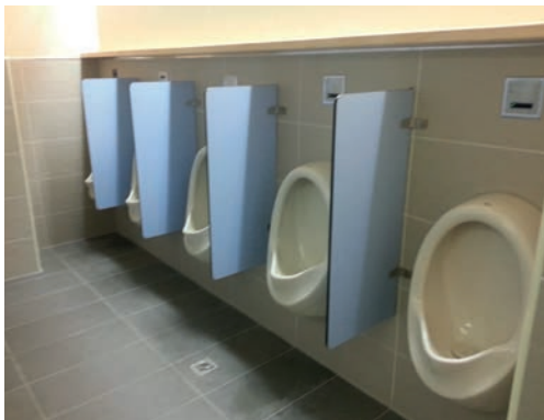
Several fixtures are discharged into Sanicubic 2 systems
