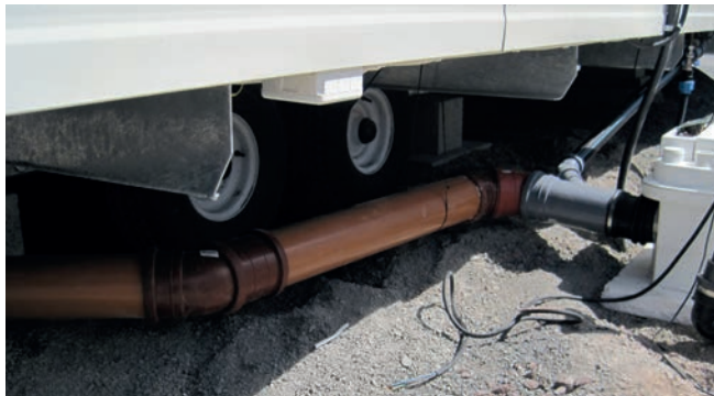
Grinder pump and alarm system protected from weather conditions
