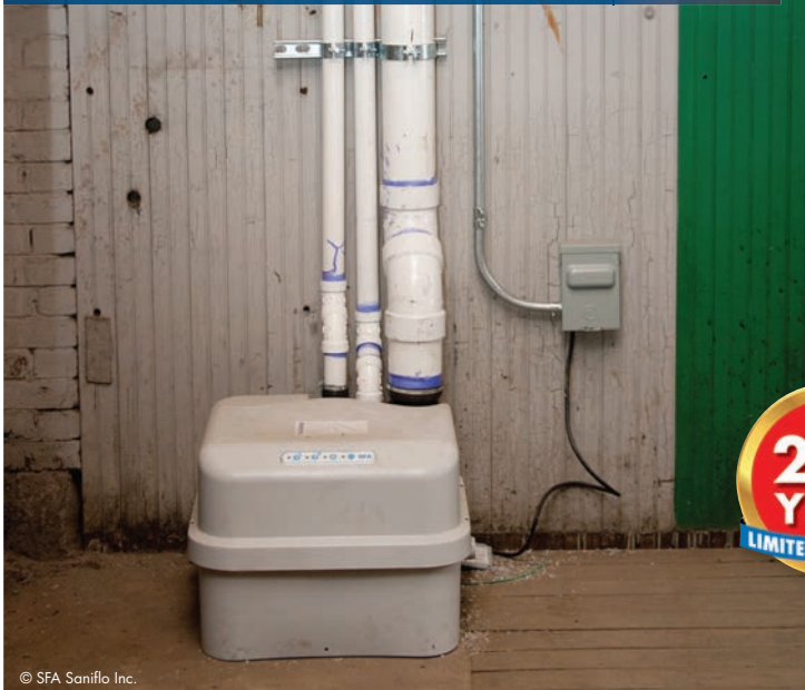
INSTALLATION ABOVE THE GROUND
