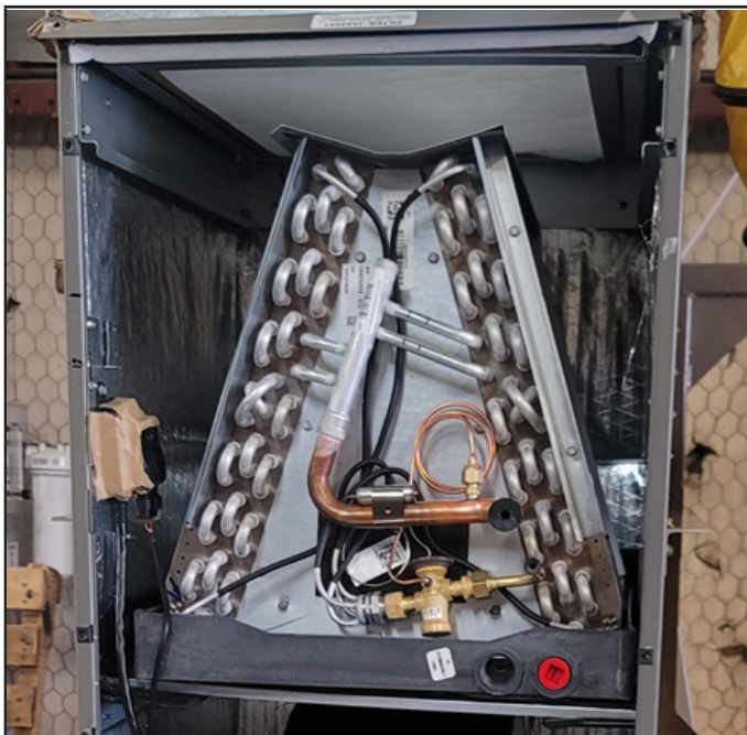
FIGURE 19. Drain Pan after Conversion
