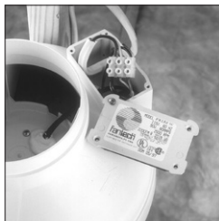
Romex wiring – Top View
