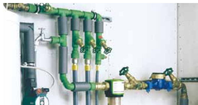
House connection station
